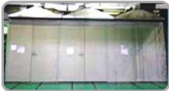
Drying room (건조로) 3 x 3 x 3(m): 3 set
