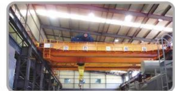
Crane (50Ton + 20Ton)
