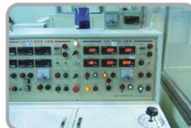
Induction voltage test (415hz)
