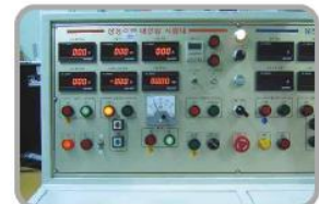
Applied voltage test (200kV)
